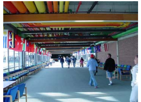
Colorful pipes in the ceiling at Utah Valley State
